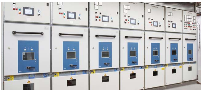
Medium voltage power distribution
