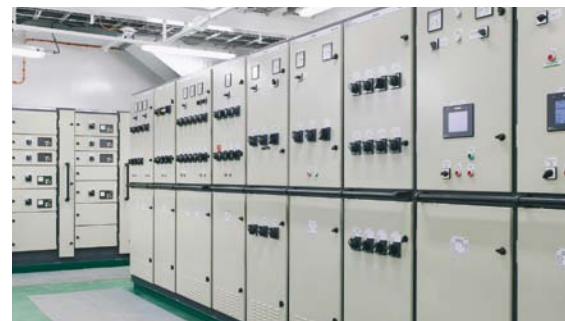
Low voltage power distribution
